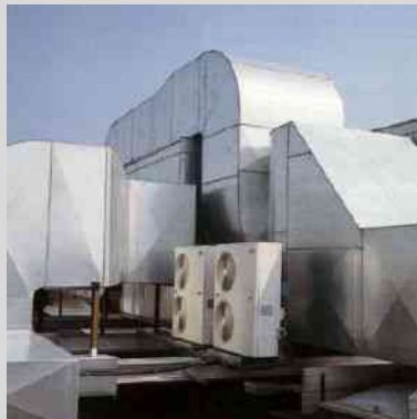
air conditioning ducts on roof
