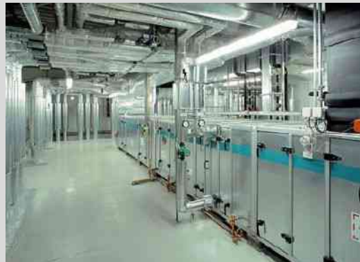
air conditioning system
